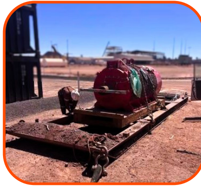
The age and deteriorated state of the previous frame was visible, showing the impact of the harsh environment.
