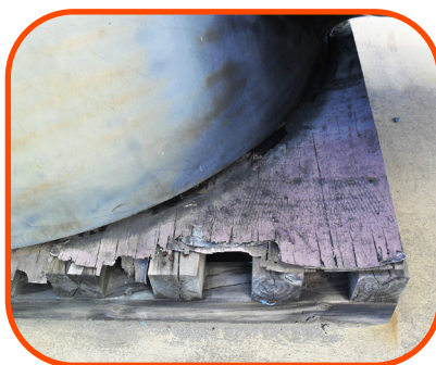
The deteriorated state of the timber was visible, showing the vulnerability of the material.
